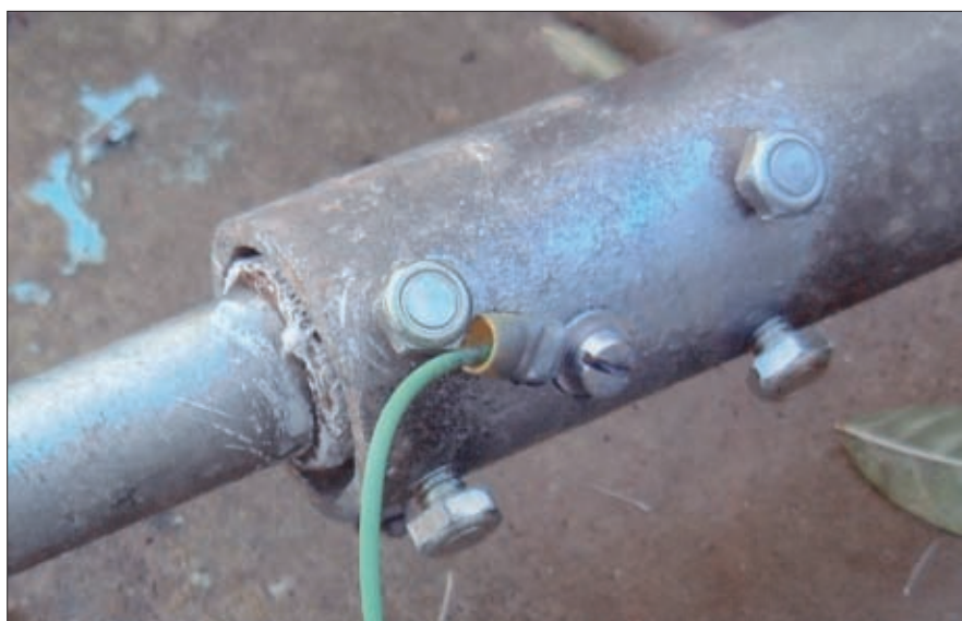
● Fig. 2: The alloy joining tube fitted into the top of the scaffold pole, using four clamping bolts. The alloy tube has been strengthened with wire mesh and car body filler.
