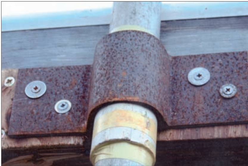
● Fig. 3: The support 'saddle' around the lower section of the scaffold pole, has a short section of plastic water pipe fitted around the pole to act as an insulator with pvc tape holding it in place.
